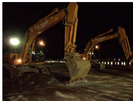
Mick Russell and Michael Garmson, both using two of our new CASE 210's, removing the deck surfacing during the closure
