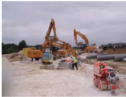
Works underway on the drainage, showing a range of the plant we utilised at the scheme
