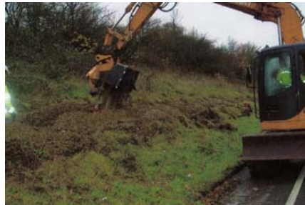
R&W's trencher unit, mounted on the CASE CX135, operated by Matt Edmunds
